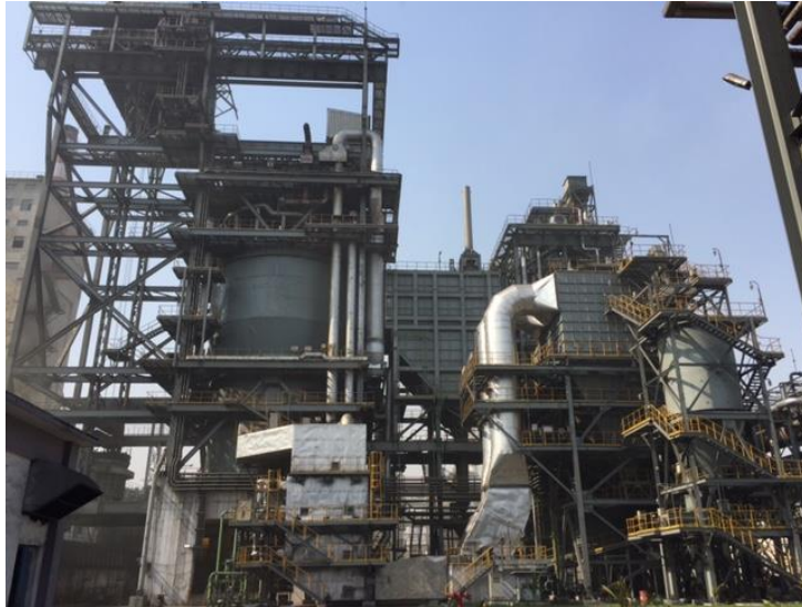
[CDQ system installed in phase1 expansion project]
