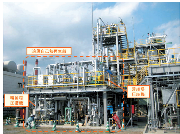
図9 自己熱再生型酵素回収蒸留設備(写真) Fig. 9 Facility of Ethanol Distillation with Enzyme Recovery and Self-Heat Recuperation (Photo)
